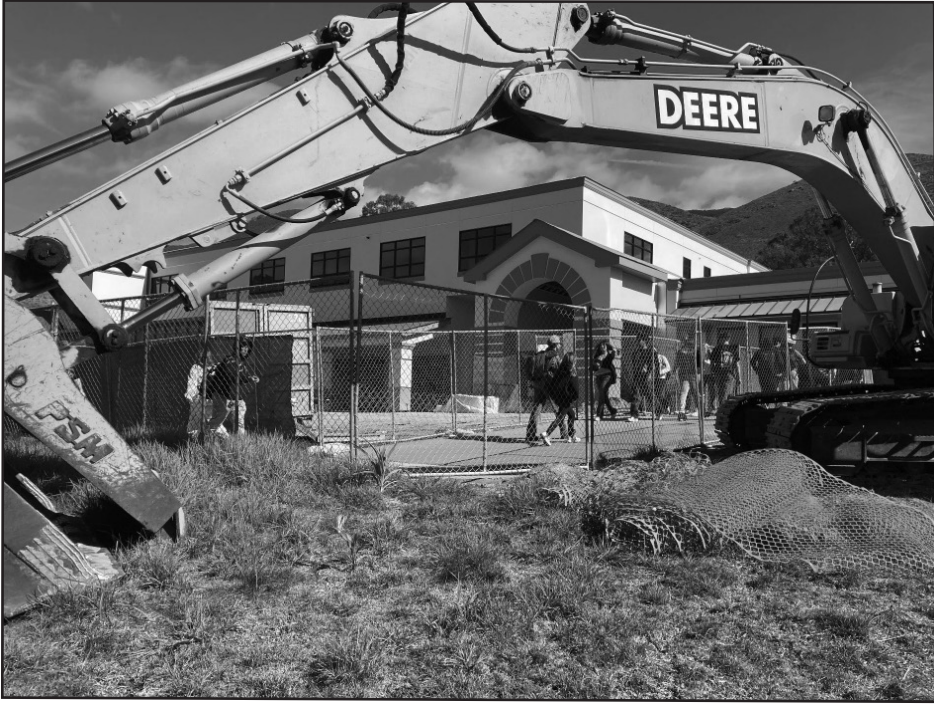
Students wind through the cafeteria construction. Photo courtesy of freshman Nico Aebischer.
